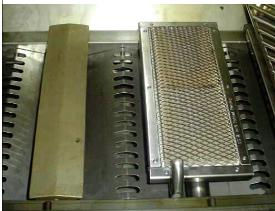
One Sear Zone burner installed
